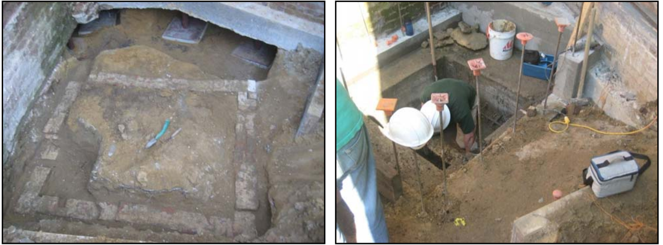
Figure 8: Privy foundation exposed during construction; work area after installation of shaft foundation
